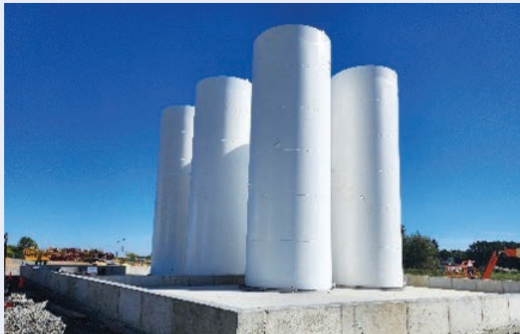
6 – 30,000 gallon tanks - expandable to 12 tanks
