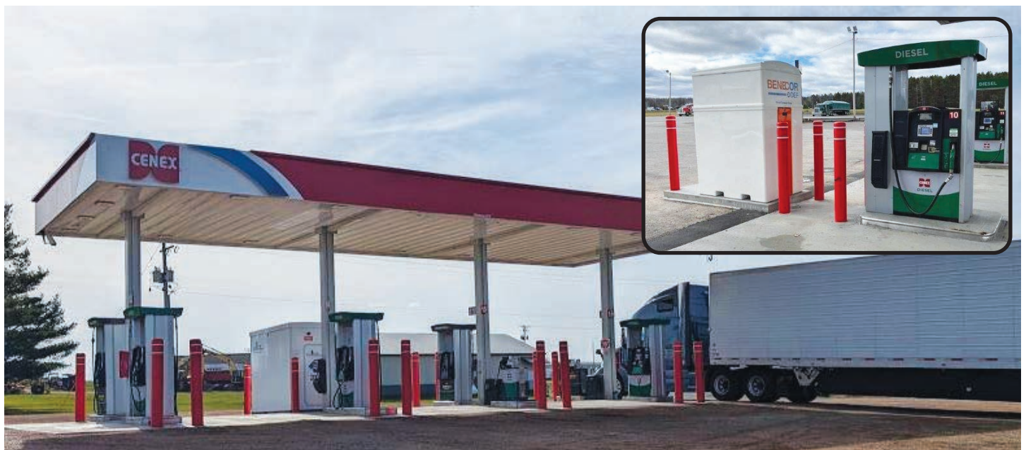
Edgar and Dorchester C-stores - DEF pumps added at the diesel islands at each location
