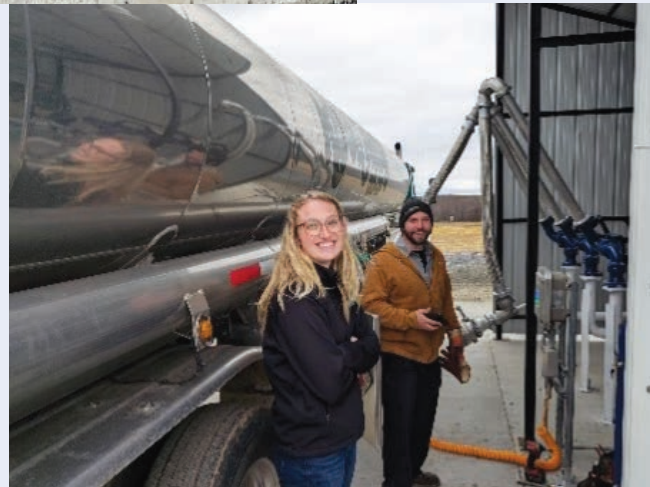
Ciara and Tim demonstrating new loading and inventory management at the new Athens fuel depot
